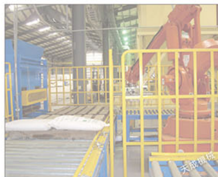
棧板供應機十堆棧設備 Empty Pallet Supplier + Palletizing System
